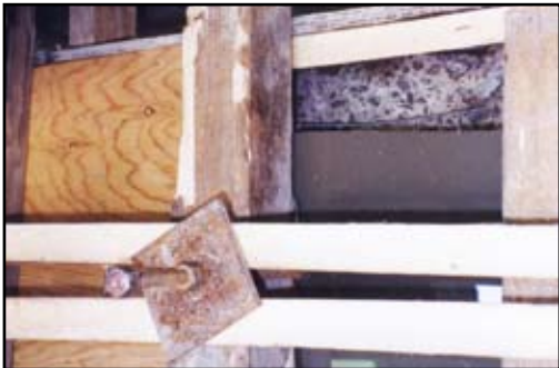
Autoroute 540/40, Quebec City, Quebec Canada. Repair of pier cap as seen through Plexiglas formwork. No internal vibration was applied. Ambex-SCC flowed freely by gravity 35 feet (11m) into formwork.
